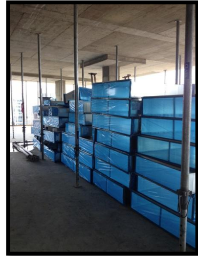
Figure 5: Duct Stored on Floor
